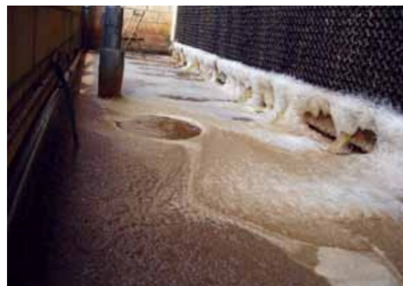
Scrubber filter before cleaning
