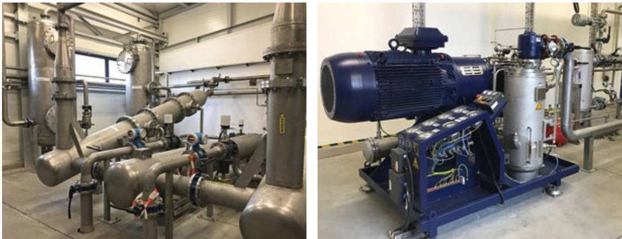
Photo 4. Biogas Purification System absorbing carbon dioxide
